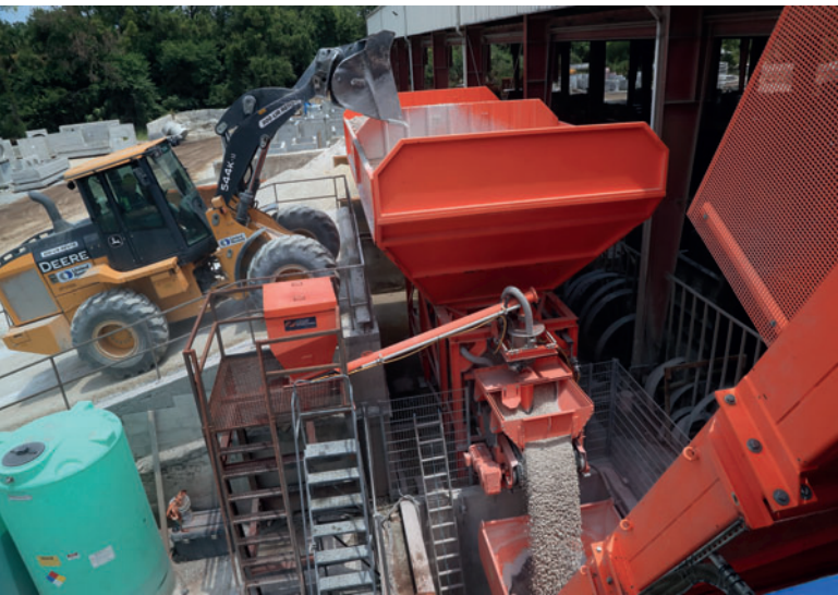
Fig 9: A front end loader refills one of two aggregate bins as the weigh belt discharges the next batch into the skip hoist bucket.
