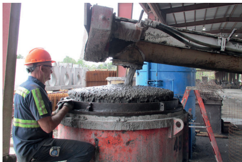
Fig 15: A form is filled on the production floor by a Tuckerbilt concrete transport vehicle.
