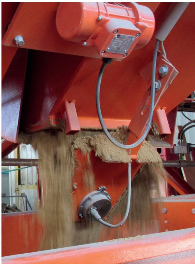
Fig 10: ACT Hydrotester moisture probe is mounted below sand bin and provides real time moisture measurement to the WCS Control system.
