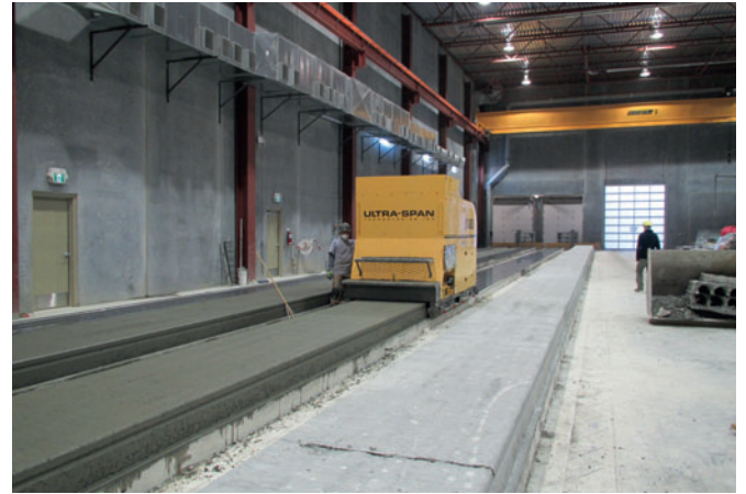
Fig. 11: Eagle Builders uses a complete hollow-core casting system from UltraSpan, featuring casting beds, dry-cast concrete extruder, saw, plotter, and hoist system.
