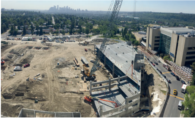
Fig. 6: One of Eagle Builders' commercial projects is a 2,000-car parking garage at the Foothills Medical Centre in Calgary. The project features a wide range of Eagle's precast products, including insulated wall panels, double tees, columns, stairs, architectural cladding, hollow-core floor and roof panels, and prestressed beams.
