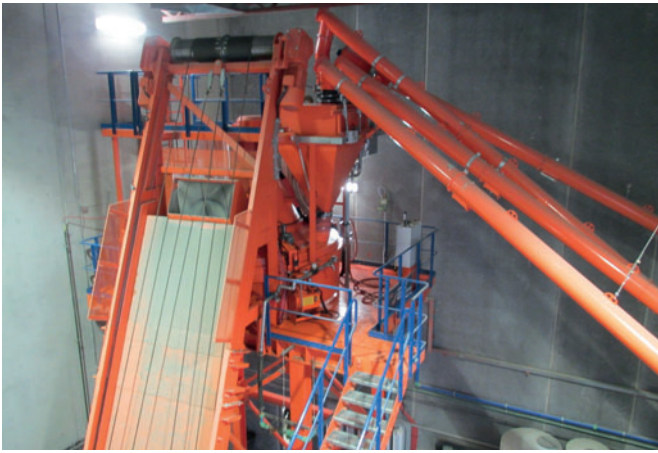
Fig. 12: The newest concrete batch plant installed at the Eagle Builders plant in Blackfalds, Alberta, Canada, features an ACT/Wiggert HPGM 4500 planetary countercurrent mixer that can produce 4 cubic yards every three minutes.
