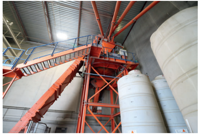
Fig. 13: Admixture tanks (right) are located at the base of the mixer platform. Eagle Builders uses Type I and Type III Portland Cement, as well as fly ash, and silica fume in its high performance SCC and dry cast mixes. Multiple cement screws (top of photo) meter into a cement weigh batcher situated above the ACT/Wiggert planetary mixer.
