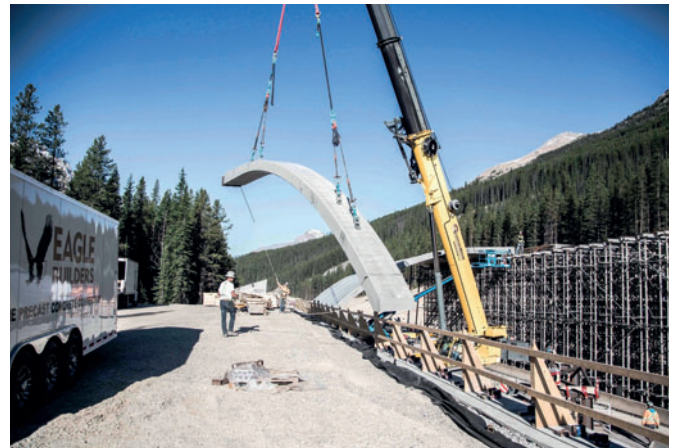
Fig. 5: Eagle Builders hoists into place one of the 100 precast arches it manufactured for one of the world's largest wildlife crossings, located in the in the Yoho National Park in British Columbia, Canada.
