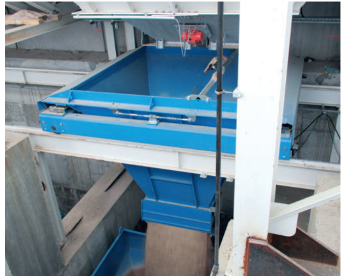
Fig. 6: An ACT/Wiggert traveling weigh batching system collects and weighs aggregates before dispensing them into one of two skip hoists, which lifts the load to its associated mixer.
