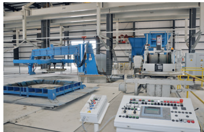
Fig. 12: The command pedestal for the Topwerk, Prinzing-Pfeiffer Variant 4000 E dry-cast machine is shown in the foreground.
