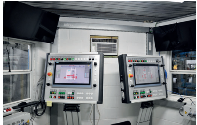
Fig. 14: Controls for both Radial Press systems are consolidated in one command center for single operator control.
