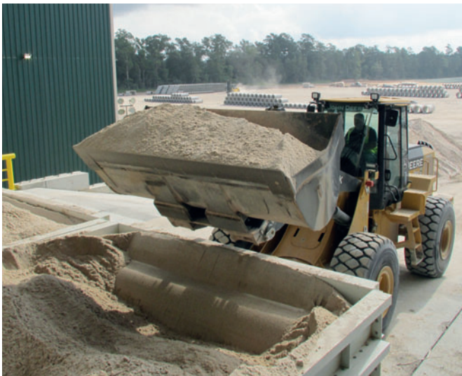
Fig. 5: A four-compartment aggregate storage system holds up to 400 tons and is filled via front-end loader. Here, sand is loaded into one of the storage bins.
