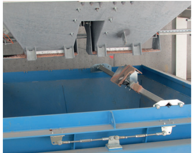
Fig. 10: Here, the weigh batching bucket (in blue) stops below one of the aggregate bins. The device mounted across the bucket is an ACT/Wiggert Hydrotester probe that measures the moisture content of every aggregate and automatically compensates batch weight for aggregate moisture measurement. Moisture is measured by a HydroMat probe in the mixer to automatically compensate for measured moisture content in order to maintain water/cement ratio that the user has defined in the concrete recipe.
