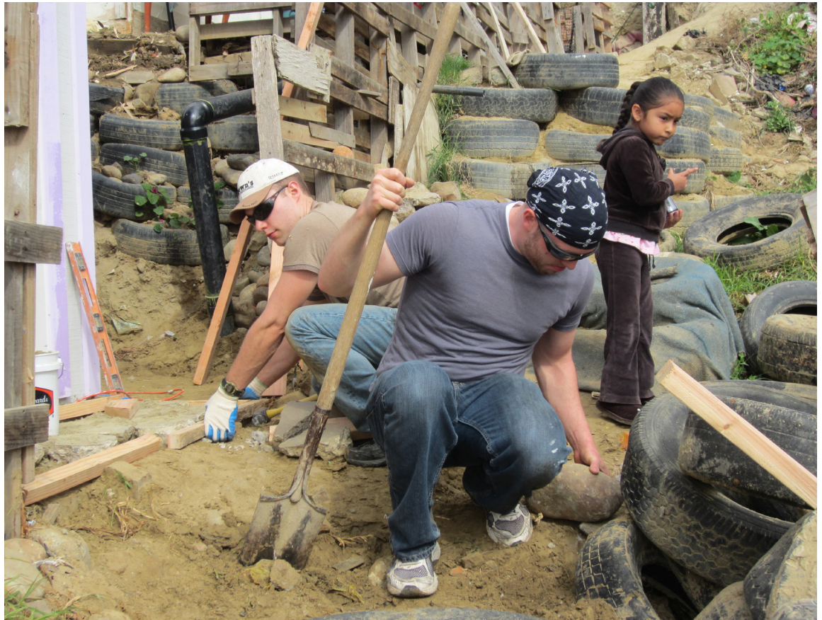
Adam Herold of Brown's Concrete and Andy Manthei of Rosetta Hardscapes build the front stoop and stairs.
