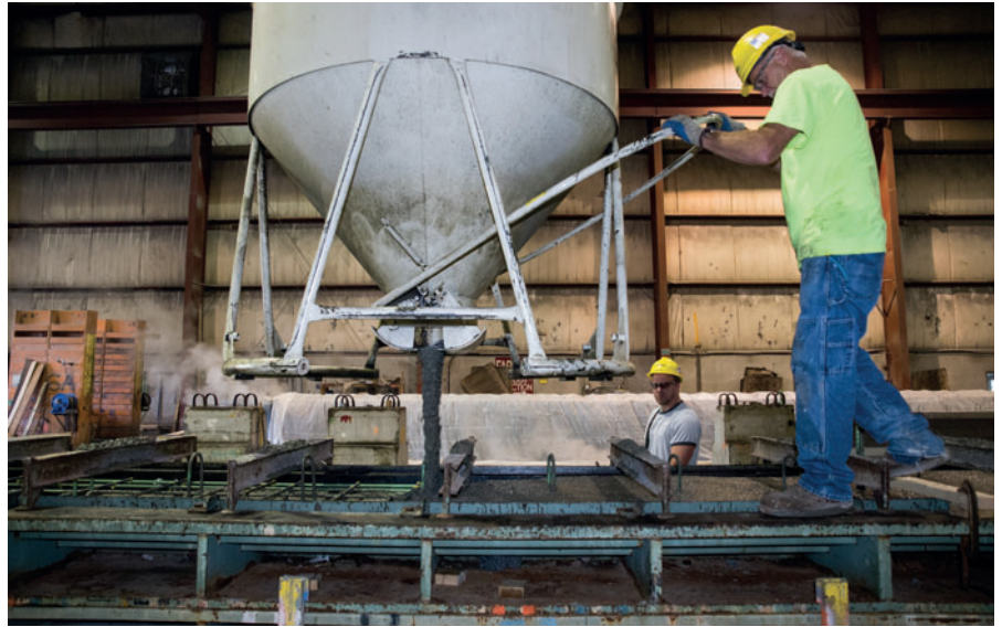
A crane bucket is used to place high performance concrete in a form on the production floor at PennStress in Roaring Spring, Pennsylvania, USA. The company transitioned in the summer of 2015 from an all ready-mix operation to an ACT/Wiggert in-house concrete batching system. Since that time, the company has seen improvements in concrete consistency, far less deviation in compressive strength, better product quality, and a significant reduction in production costs.
