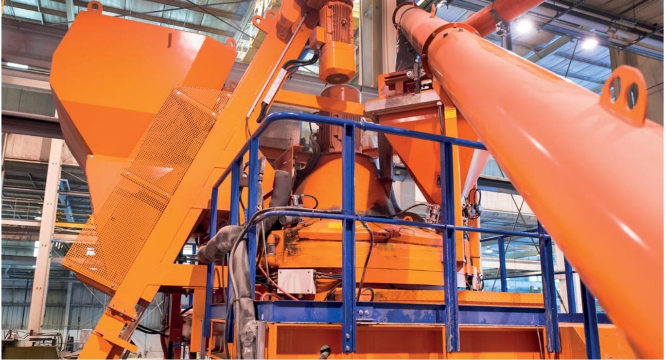
One of two mixer platforms, each equipped with an ACT/Wiggert HPGM 2250 two-cubic-yard (1500L) planetary counter-current mixer, receive aggregates from a skip hoist (left) and cement and fly ash screws (right). Each mixer is equipped with two discharge gates, one for dry cast and one for wet cast and clean out using an automated high pressure mixer cleaning system.
