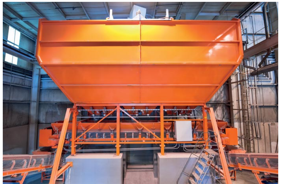
Jessup batch plant installation includes a low-profile 195-ton three-compartment aggregate storage system, including weigh belt conveyor, from ACT/Wiggert. Hydrotester moisture sensors located below each aggregate bin, combined with microwave probes in each mixer, enable the PCS control system to consistently and accurately maintain the correct water/cement ratio for every batch.
