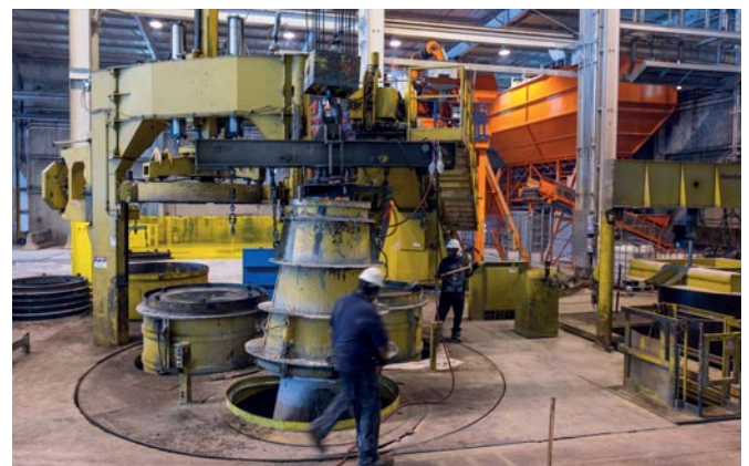
The outer mold for a flared-end pipe is lowered into position on the HawkeyePedershaab PipePlusPlus precast production system. In the background, a worker tends to a newly cast 60-inch precast pipe in preparation for its rotation into the pressheading station. The PipePlusPlus system allows multiple products to be produced simultaneously to match customer needs. The PipePlusPlus and other production stations in the CP&P Jessup facility are supplied with fresh concrete by the ACT/Wiggert batching system.
